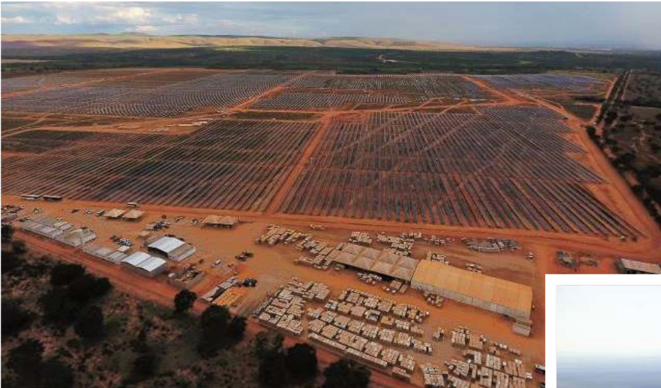
UFV de 185 MWp, Pirapora (MG).
